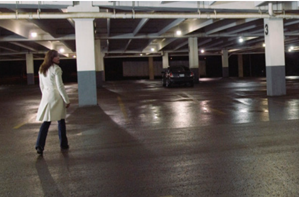
Entire floors are ignited to full power to deliver an added sense of security.
